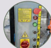
Electric control system
